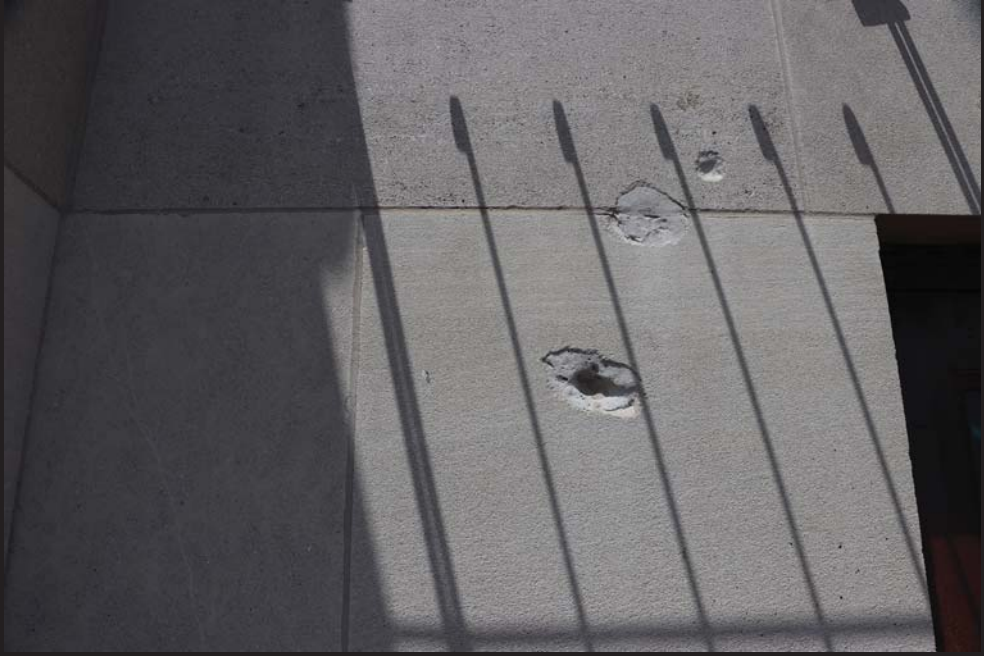
FIGURE 9.3 Bullet Holes atop the Tower
