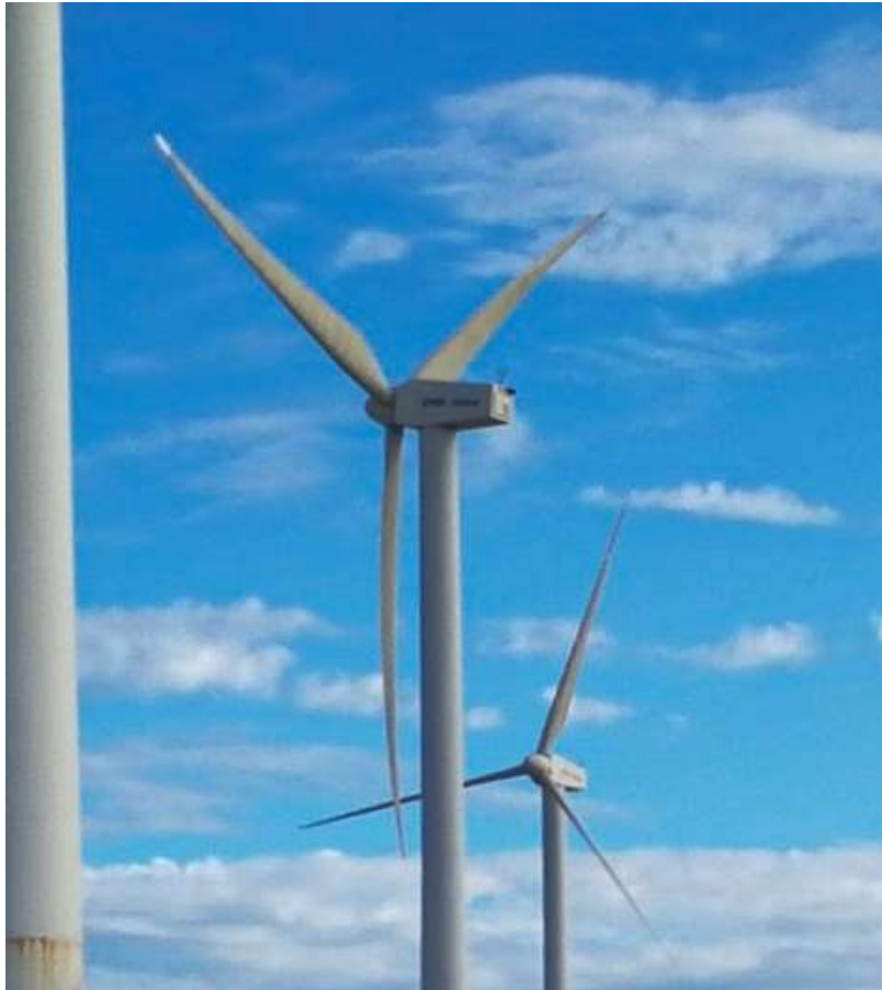
Wind turbines, Gibara
