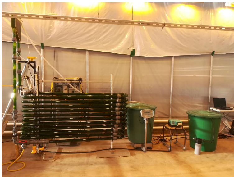
Figure 5. The tubular photobioreactor operation installed in the greenhouse.
